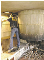
A volunteer works around the fireplace in the Spring House during a cleanup of the Frank Lloyd Wright-designed home on Jan. 12. GERALD ENSLEY/DEMOCRAT
